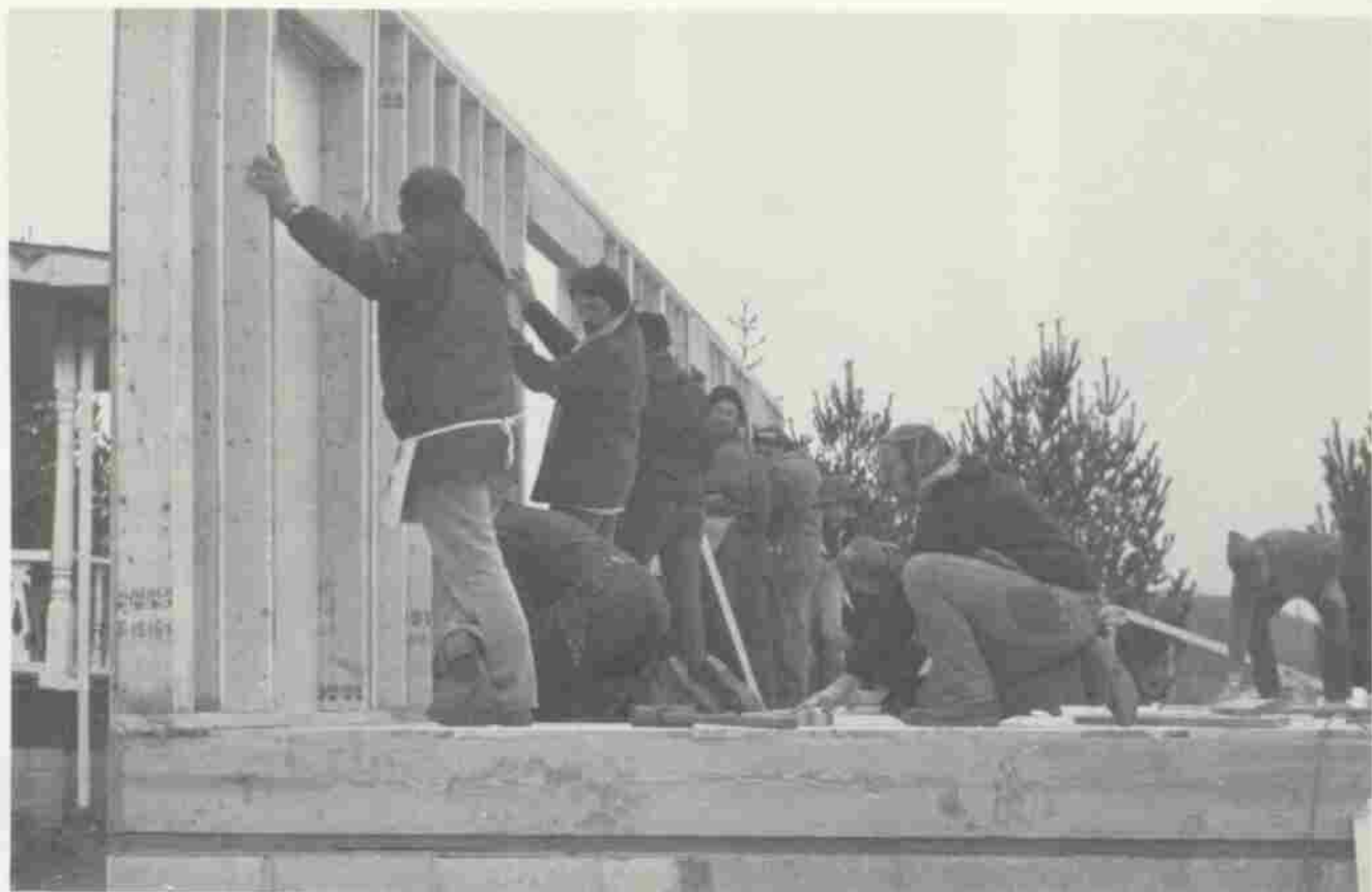
Many of the teachers helped to rebuild the home of Mr. Smith, which burned December 20, 1982. Mr. Meyer (kneeling) and Mr. Stoffel led the project. The picture shows the first upstairs wall being erected.
